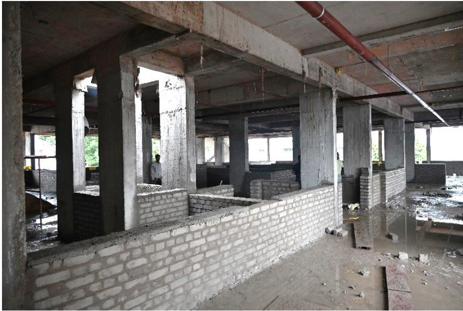
Fire safety pipework on first floor Block A
